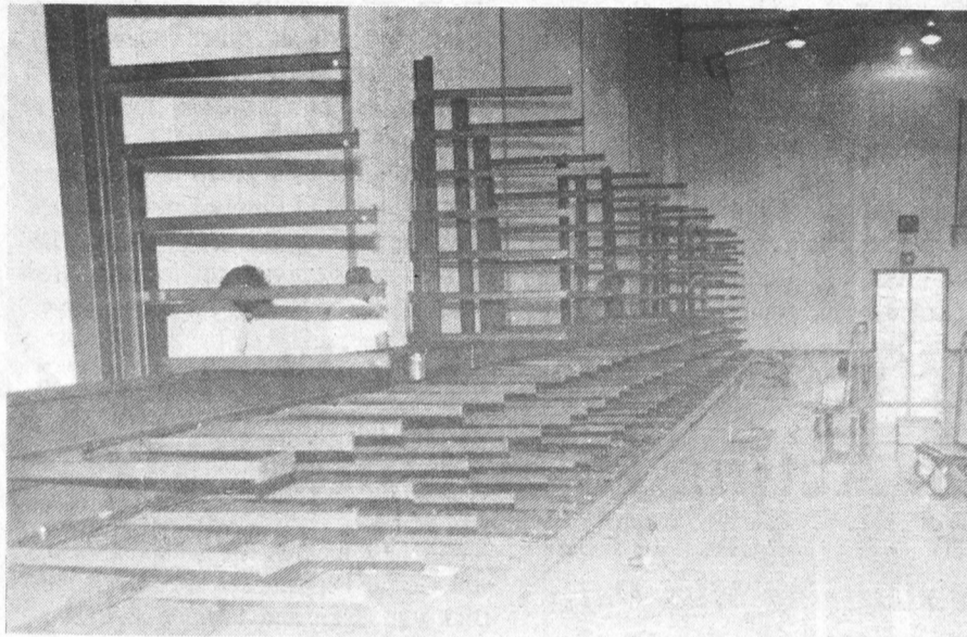
Special Photo/CSC Media Services Last month the frame for the bleachers was being installed in the gymnasium. The workers still needed to add the flooring, benches and reserved seating areas
