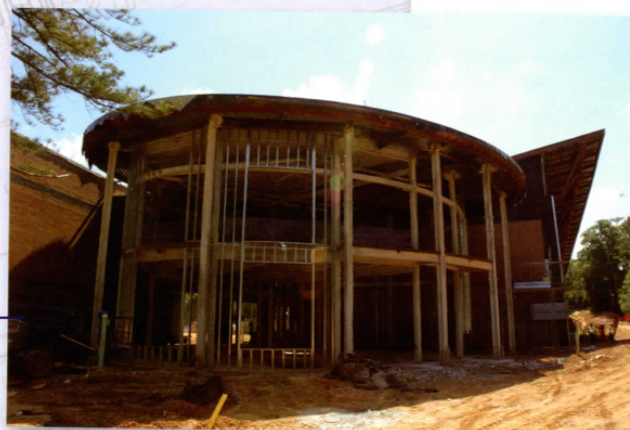
Shown nearing its completion, the Student Activities Center promises to be the new student hang out on campus.
