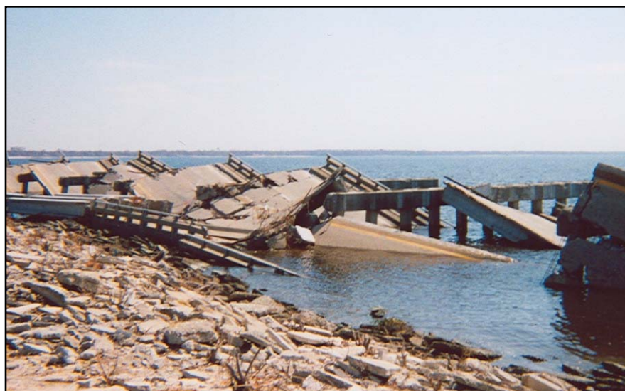
Stacey Clements, at the time a senior in Clayton State's nursing program, snapped this picture of a destroyed bridge as her group journeyed to the badly damaged Biloxi area.
